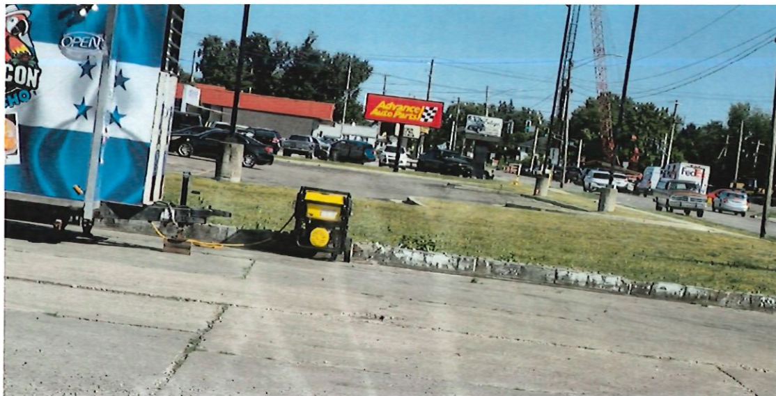
Gas generator at west end of food truck - May 28, 2026
